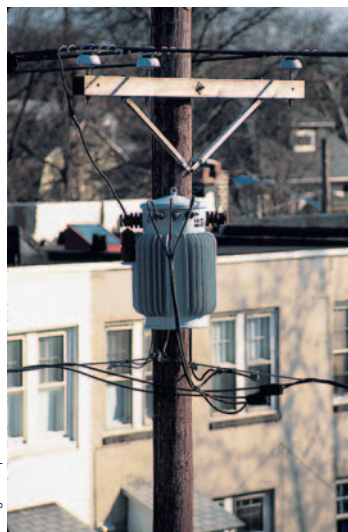
This cylindrical step-down transformer drops the voltage from 4 000 V to 220 V for delivery to a group of residences.
